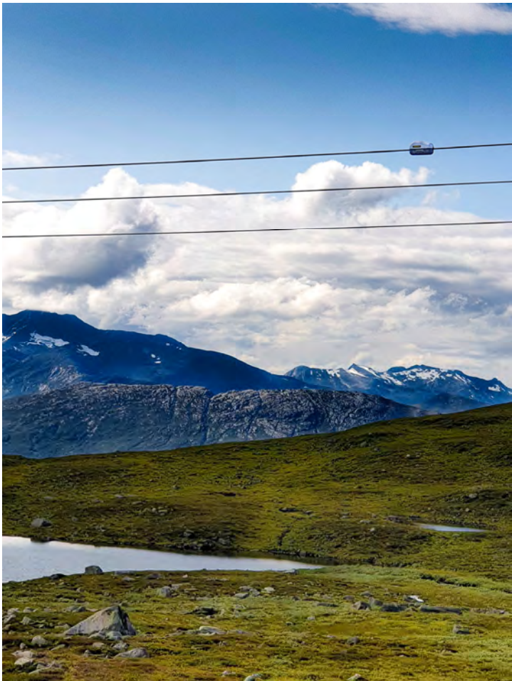
The TLM monitor uses built-in LiDAR to directly measure the distance from the conductor to the ground below. Compared to other methods that determine conductor sag, this method accurately provides the actual electrical clearance of the line.
